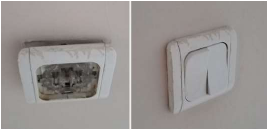
Figure 4.18 Electrical outlet fixed by P15.
